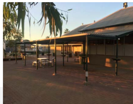
Front area paving has inconsistent levels.
