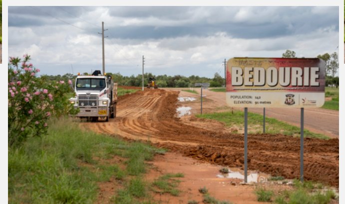
Photos: The Bedourie levee bank was raised in sections at the beginning of March as a precautionary measure.
